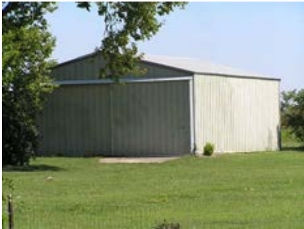
Figure 2.15: Southwest facade of the 41'x31', white, metal shed (Structure #6); this building is in good condition and proposed to become the gathering place for gardening, orchard activities and other potential indoor/outdoor programs
