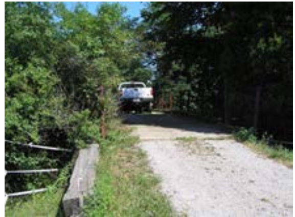
Figure 2.20: Vehicle driving over the bridge before structural inspection; the design is simple and utilitarian
