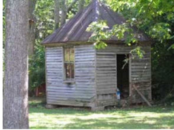
Figure 2.24: Wood construction and weathered roof give this shed character; it can be repaired with reclaimed materials from other buildings on site
