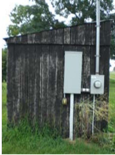
Figure 2.10: Electric meter should be removed or relocated
